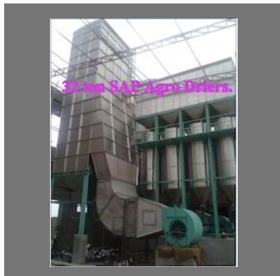
Steam Dryer Plant
